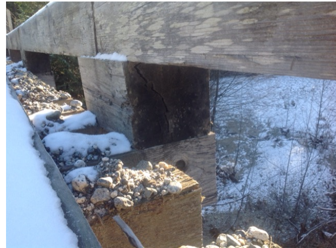
rotten and splitting risers
