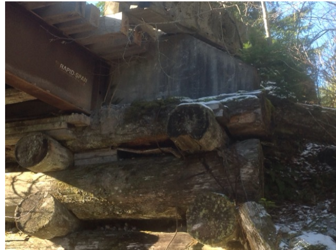
top crib log on right abutment Fd and in relatively poor shape
