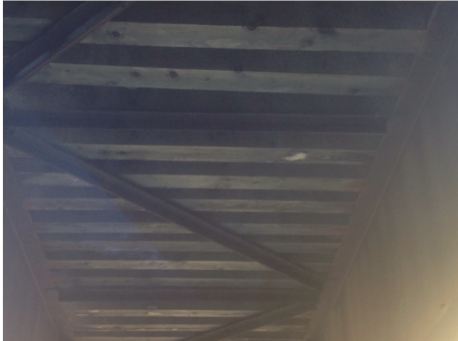
some ties in fair to poor shape
