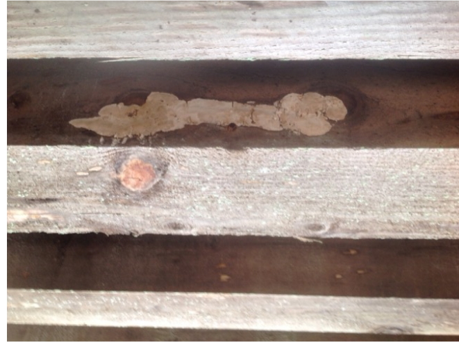
more ties that are rotting
