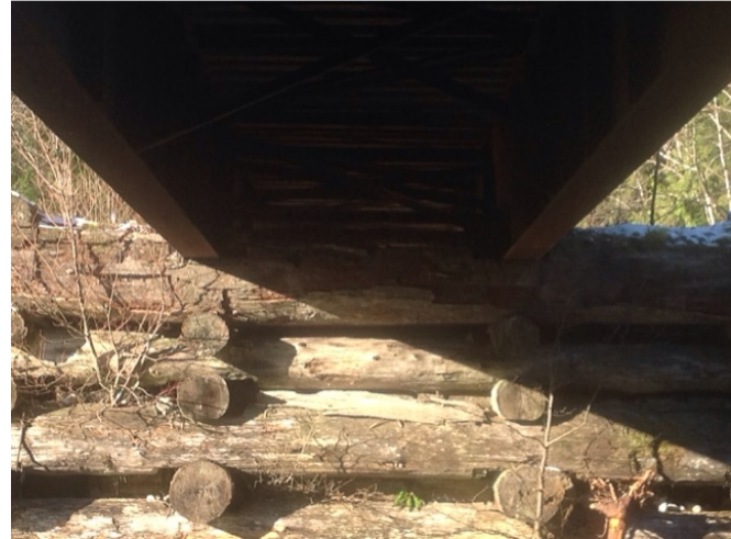
top crib log of pier, on left side in poor shape
